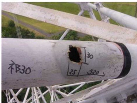
Figure 9. Pitting of a steel pipe member
