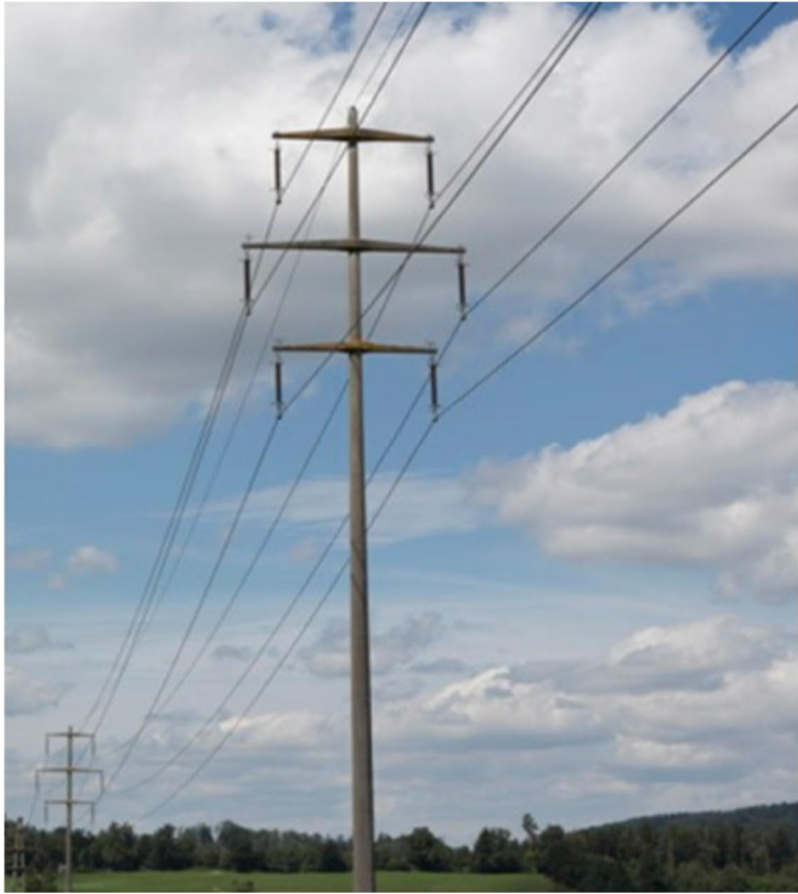
Fig. 1 View of a 50 kV high-voltage line
