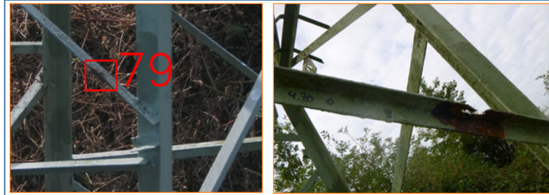
Figure 9: Same damage seen by drone (Left picture) and by climbing inspection after stripping (Right picture)
