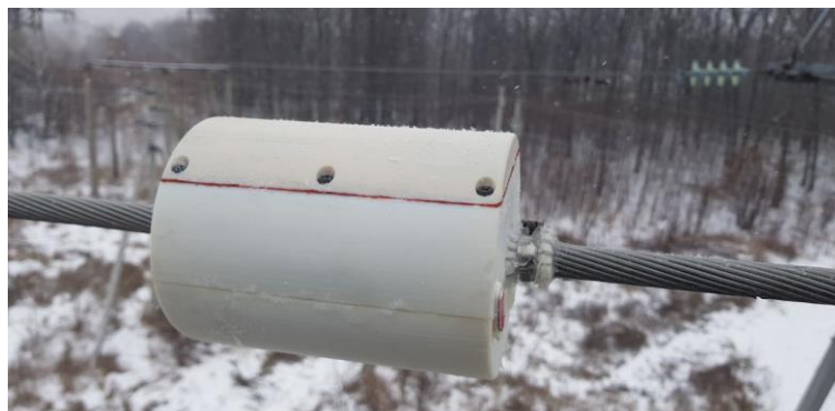
Fig. 1. Control device of the overhead line condition monitoring system installed on the conductor
