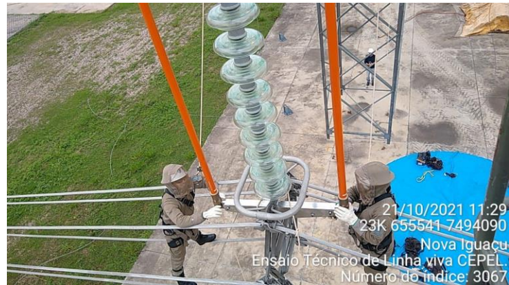
Figure 12 – Linemen performing the connection between tension sticks and the metal component for supporting the conductors
