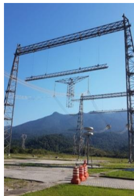
Figure 5 – Upper part of \pm 800\text{ kV} DC guyed tower assembled in the UHV laboratory
