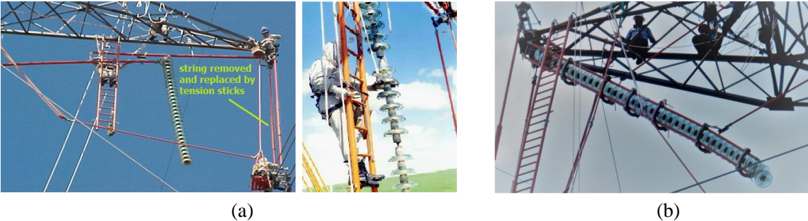
Figure 3 - Methodologies applied to replace damaged cap and pin insulators using (a) trolley pole and (b) cradle
