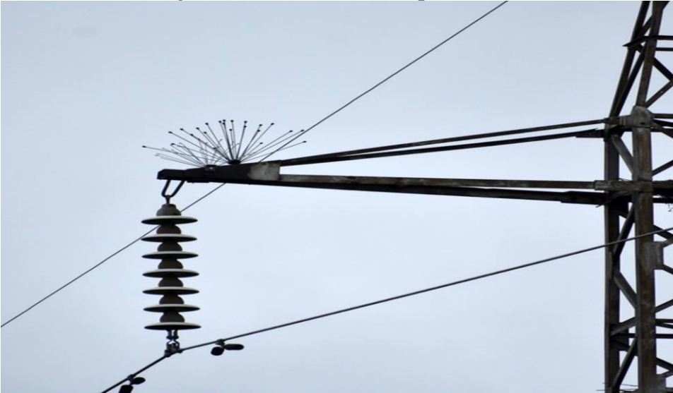
Pic 3. Anti-landing devices on the electric power towers
