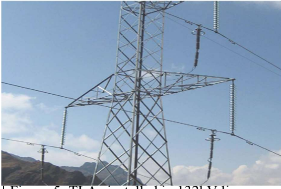
Figure:5: TLAs installed in 132kV line
