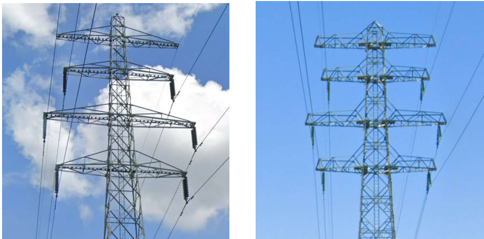
Figure 2: Cross Arms of Lattice High-Voltage Towers without (left) and with (right) Handrail
