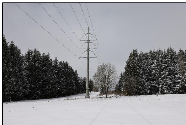
Figure 20 : Picture of a tangent pole with insulated cross-arms
