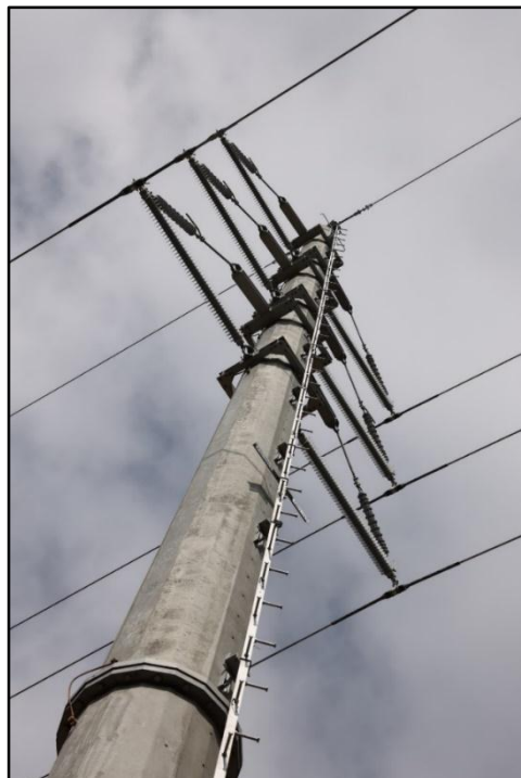
Figure 22 : Upper part of a tangent pole with insulated cross-arms
