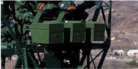
Figure 16 – Noise insulation passive shields mounted on the circuit breaker command cubicle.
