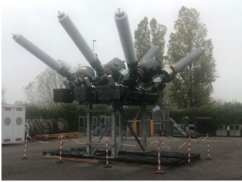
Figure 9 – HV SF 6 insulated equipment before installation.
