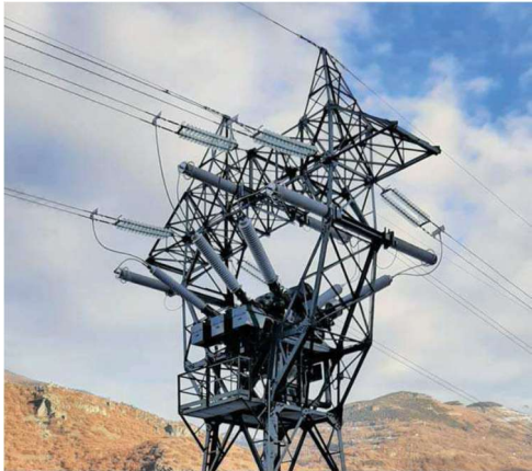
Figure 5 – HV SF6 insulated equipment on tower.
