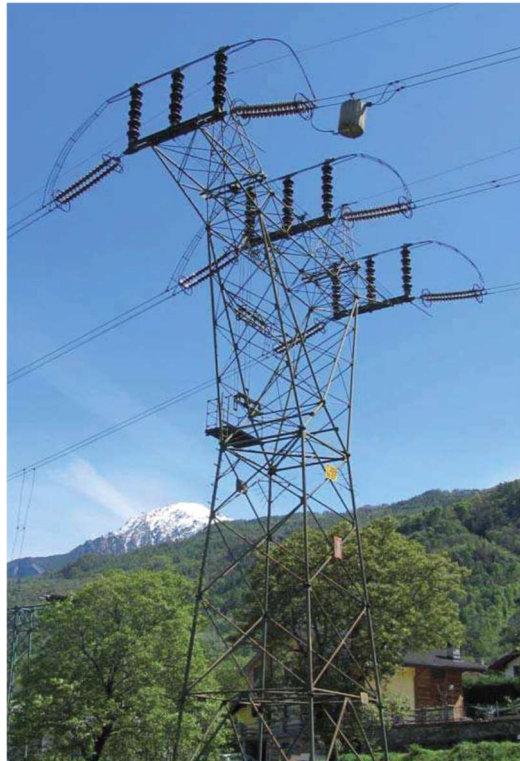
Figure 3 – Typical disconnectors installed on 220 kV “Delta” tower.
