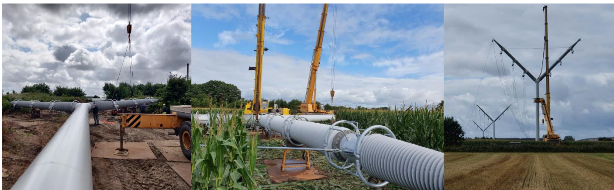
Figure 7 : Left: Preparing of installation. Middle: Cranes ready for erection. Right: Pylon installed.
