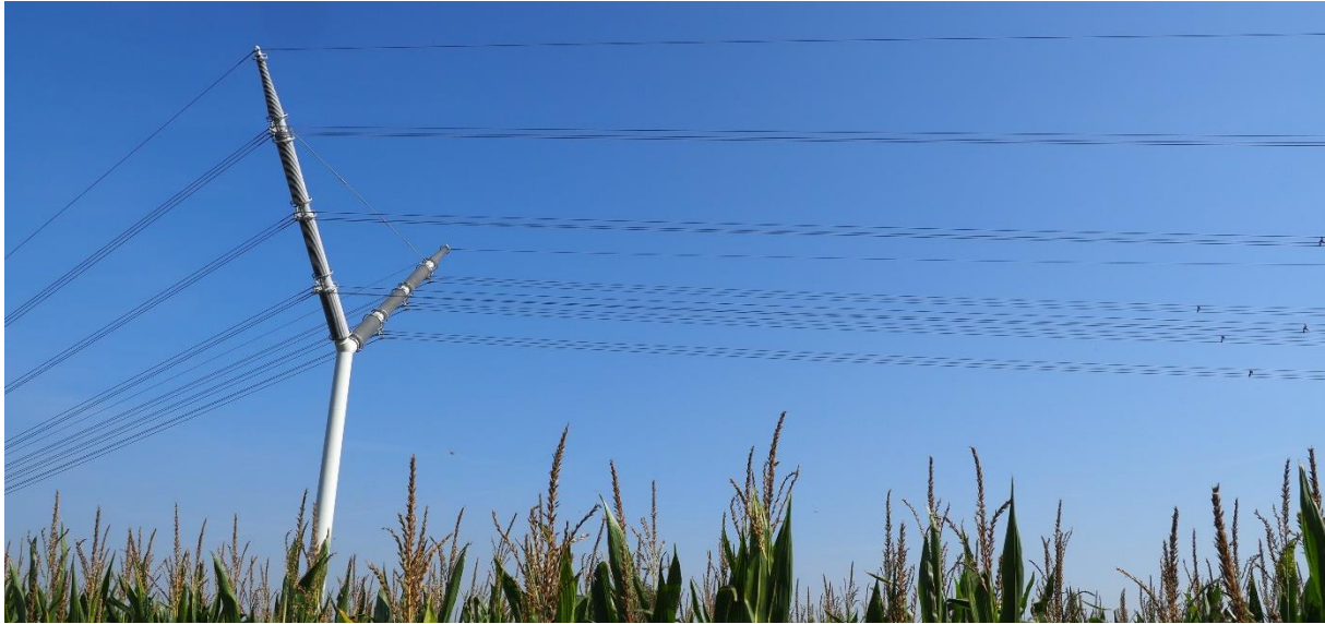
Figure 1 : Demonstrator of 400 kV European Composite Pylon
