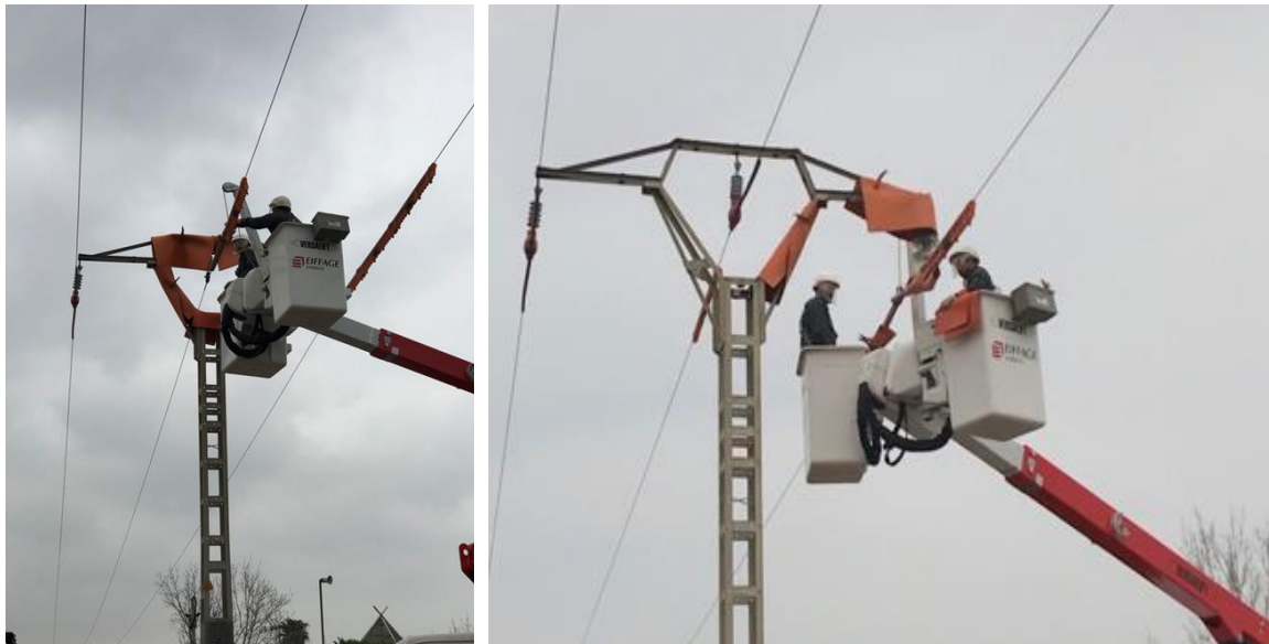
Figure 1 Example of working procedures related to case 2 Installation of avifauna protectors on medium voltage overhead lines (20-30 kV).
